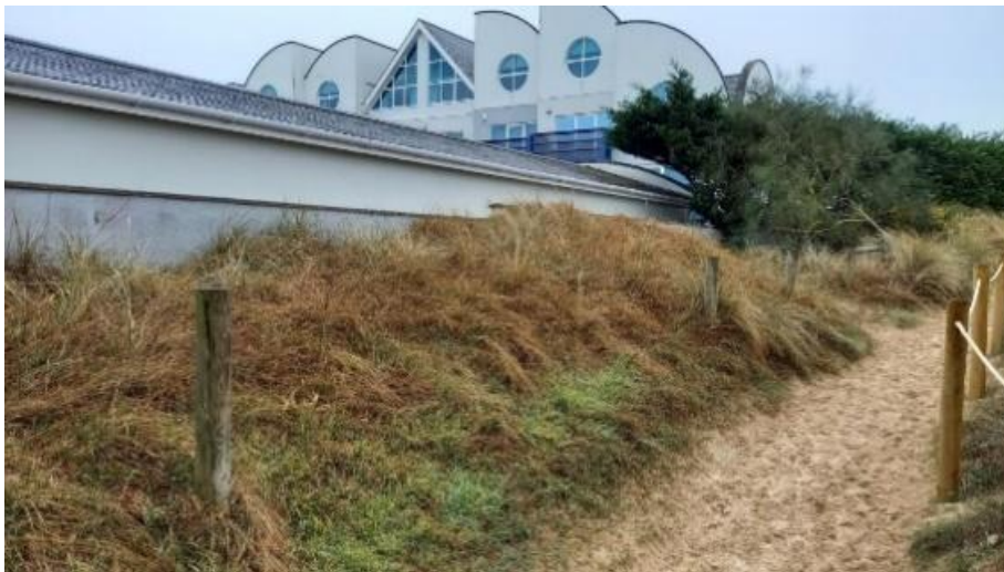
Figure 9 - Sand build-up along boundary wall at Sandbanks, posing structural stability issues.
