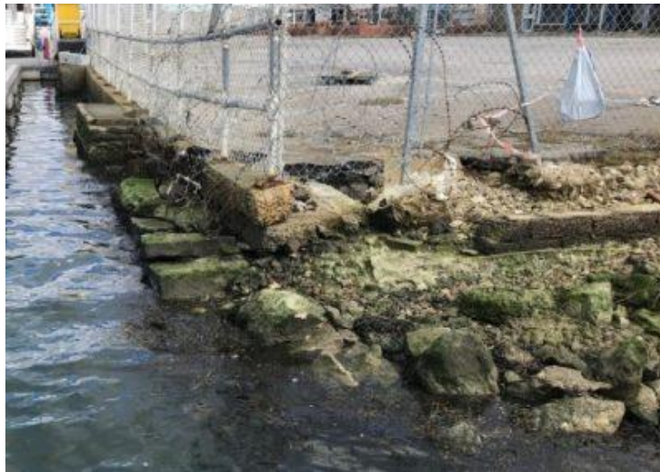
Example of the very low level and poor condition of the current quay walls.
